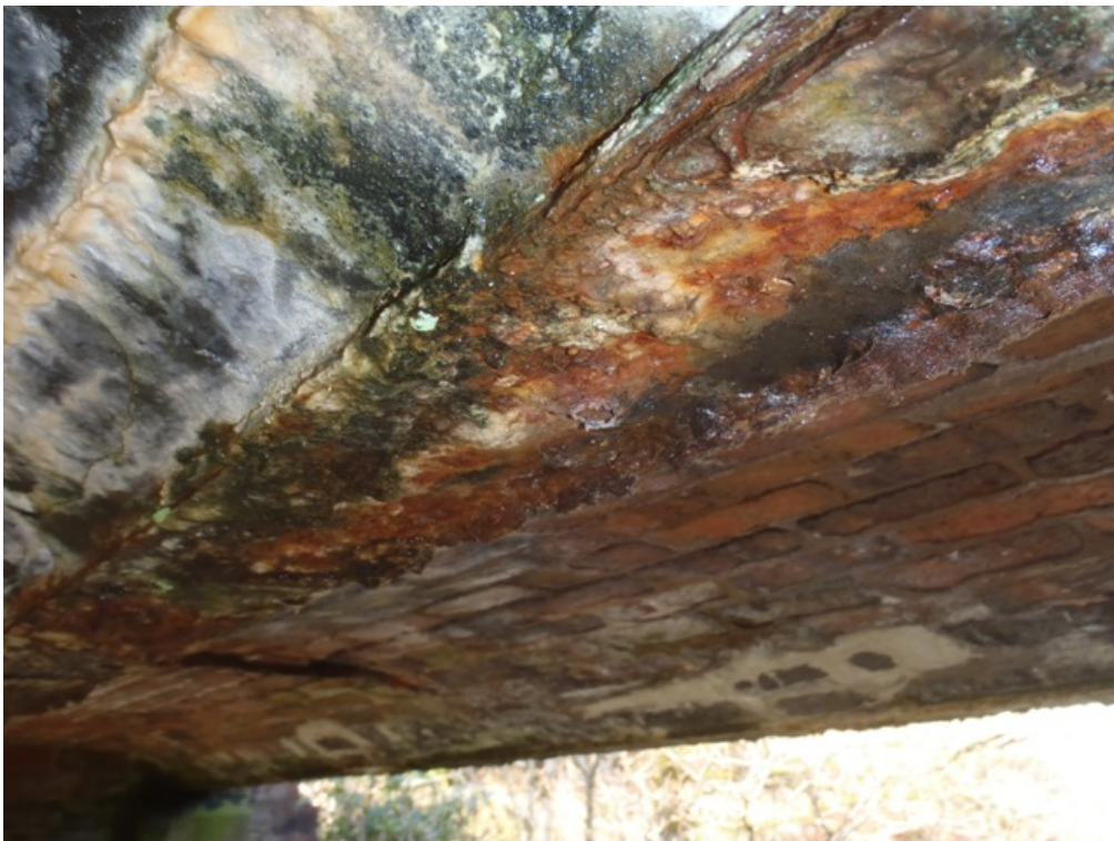
Photo 8 typical corrosion to underside of main girders 11/02/2014
