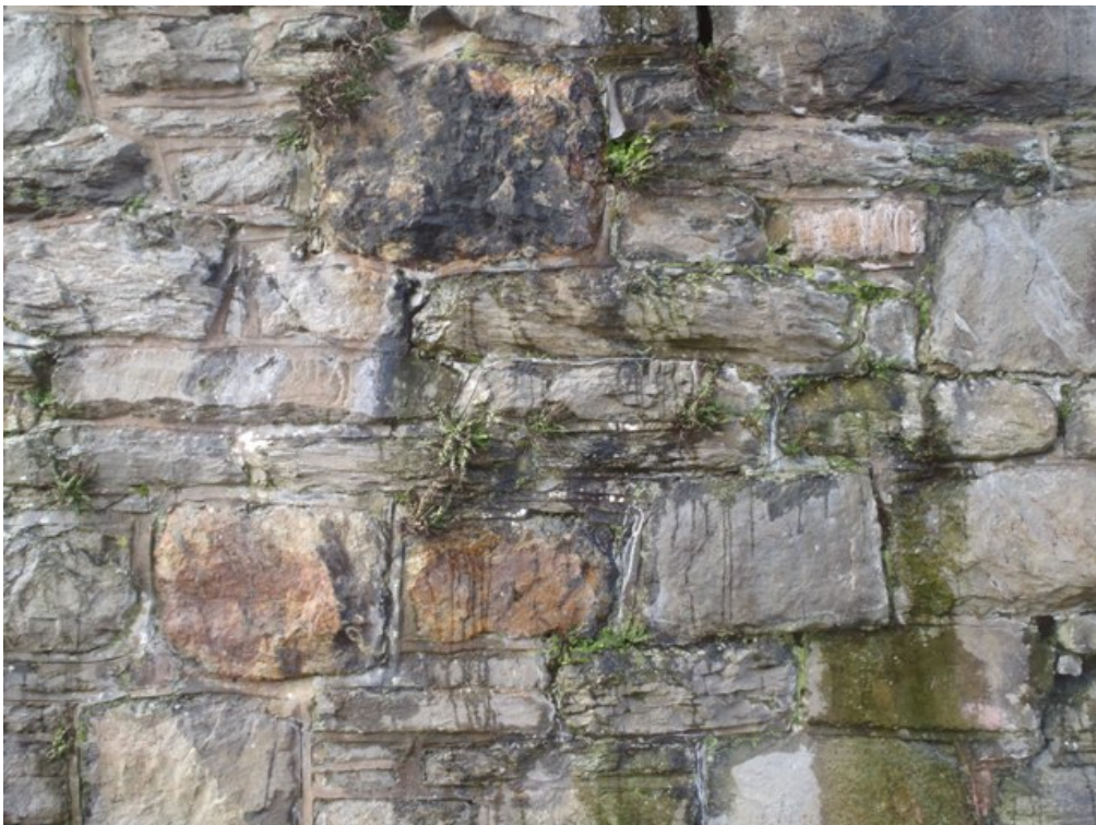
Photo 12 fracture at upside abutment 11/02/2014
