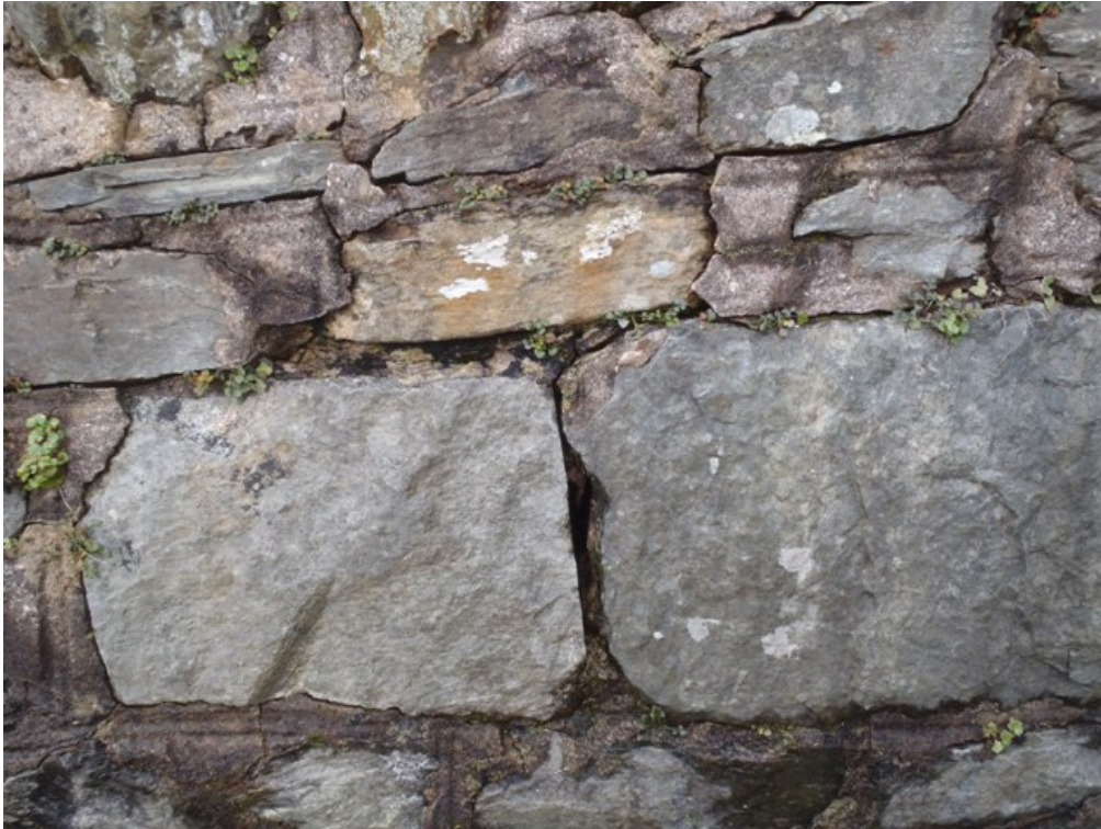
Photo 17 typical open joints at parapet walls 11/02/2014
