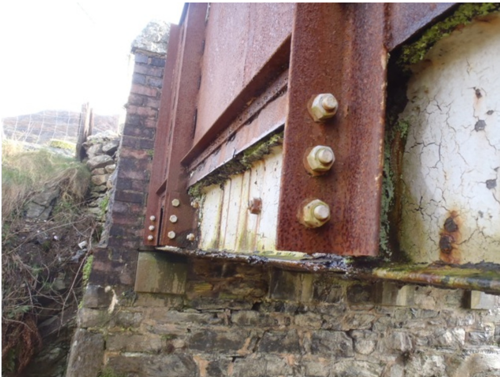
Photo 6 typical corrosion to outer main girder 11/02/2014
