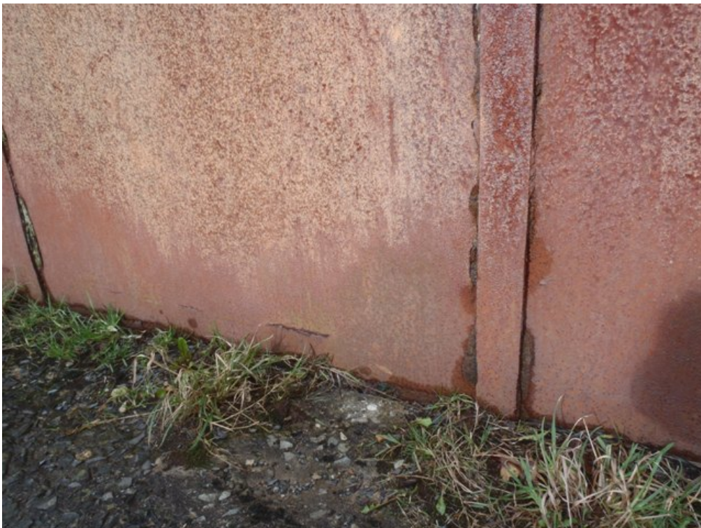
Photo 16 typical corrosion at Blaenau end parapet 11/02/2014
