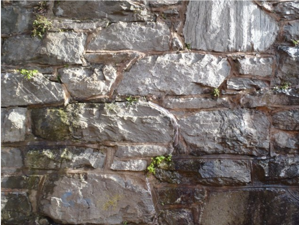
Photo 11 fracture at downside abutment 11/02/2014
