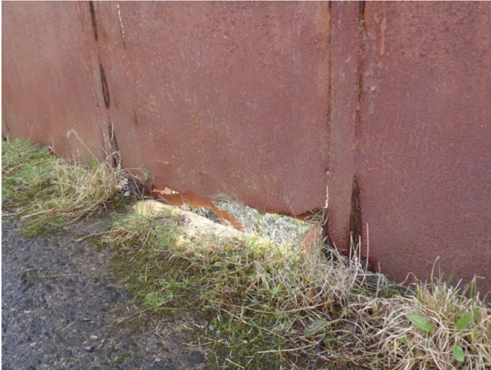
Photo 15 typical corrosion at Trawsfynydd end parapet 11/02/2014
