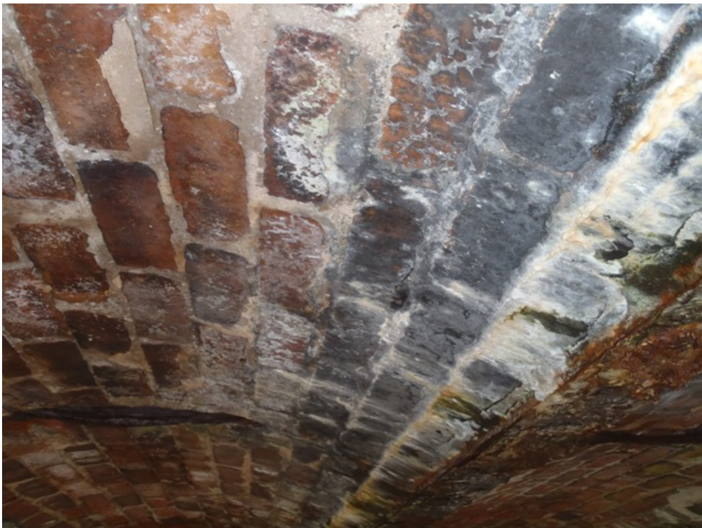
Photo 18 typical water seepage at jack arches 11/02/2014
