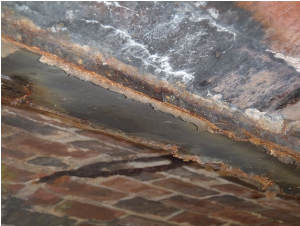
Photo 9 typical paint failure at main girders 11/02/2014
