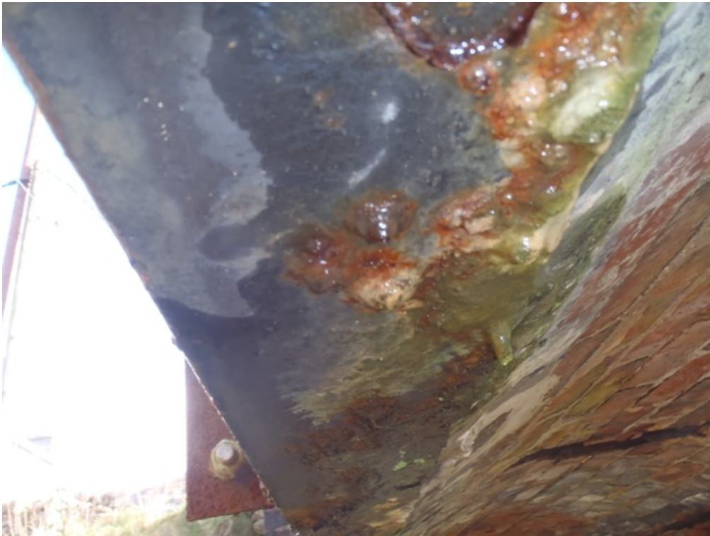
Photo 7 typical corrosion to underside of main girders 11/02/2014
