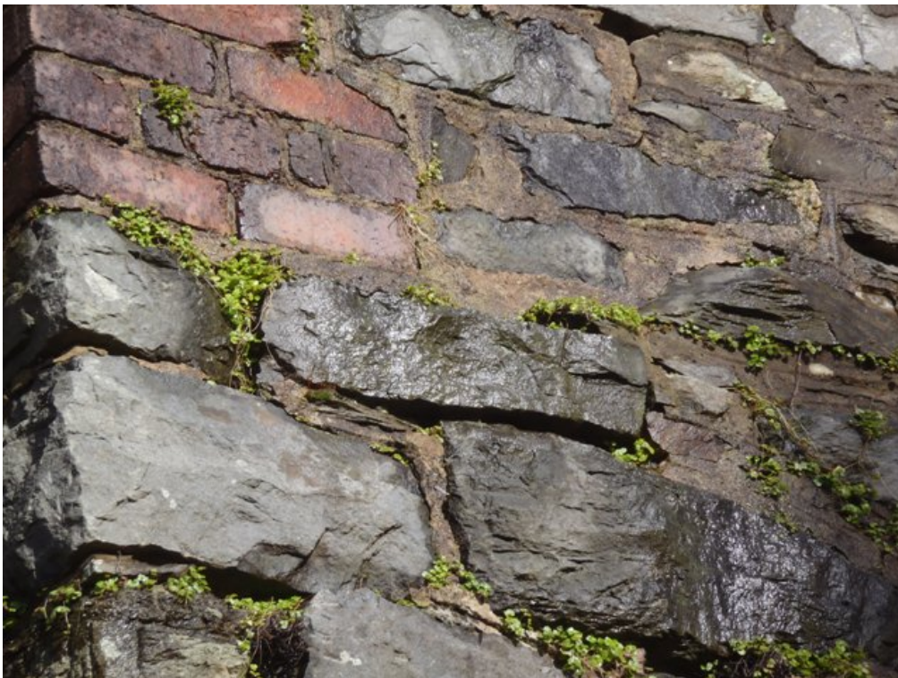
Photo 14 typical open joints at wingwalls 11/02/2014
