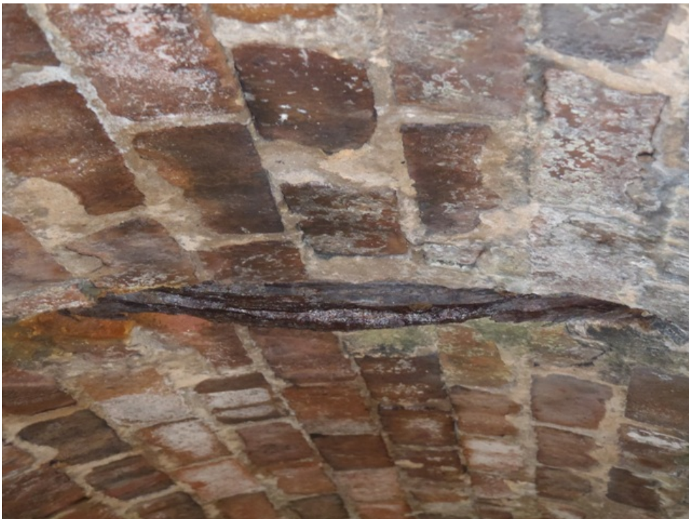
Photo 22 typical corroded tie bar 11/02/2014
