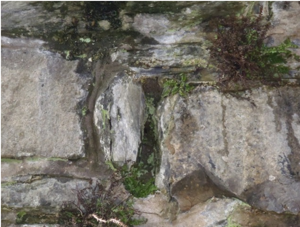
Photo 13 typical open joints at abutments 11/02/2014
