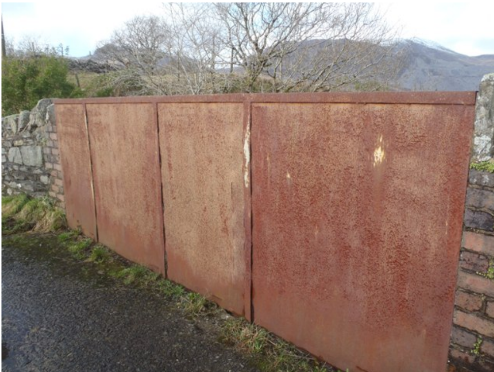
Photo 10 typical paint failure at parapets 11/02/2014
