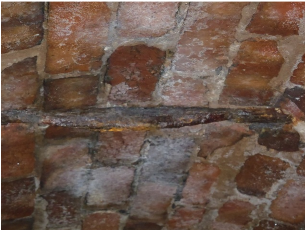
Photo 24 corroded tie bar 13/02/2014
