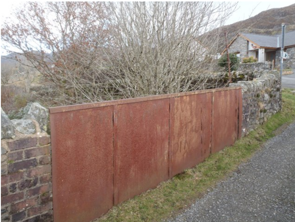
Photo 20 typical paint break down at parapets 13/02/2014
