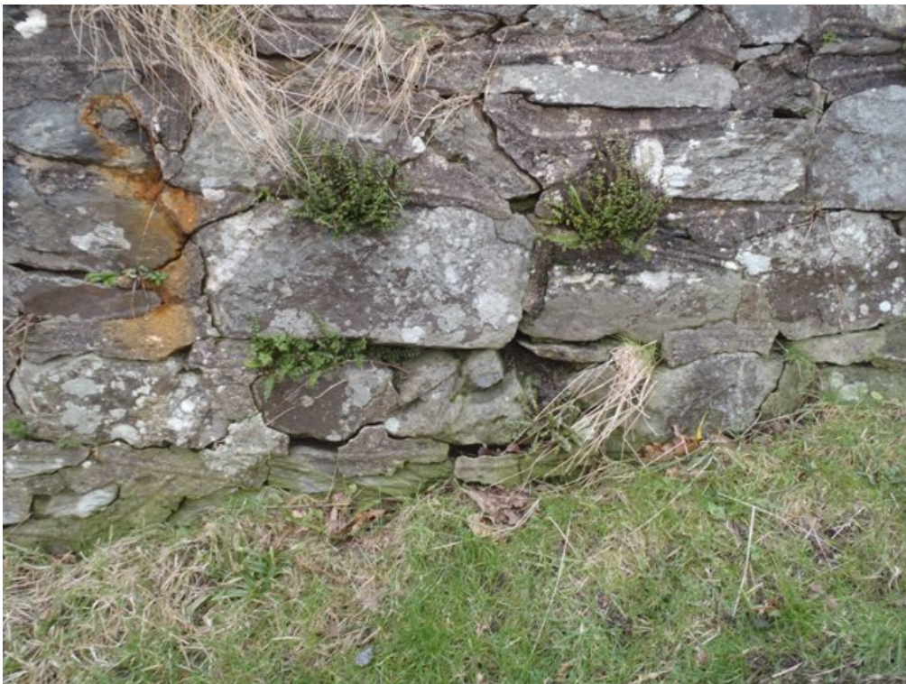
Photo 16 typical open joints at parapets 13/02/2014
