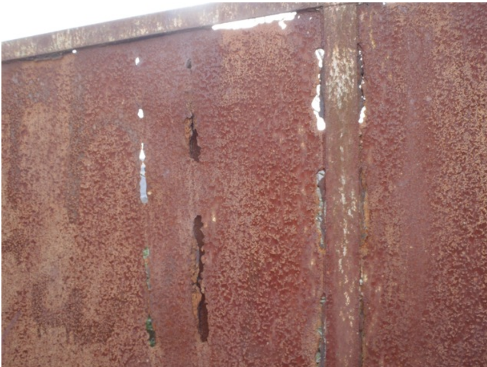
Photo 14 corrosion to Blaenau end parapet 13/02/2014
