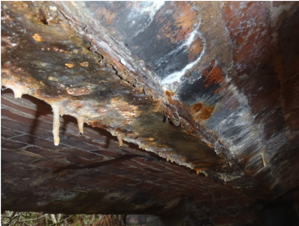
Photo 7 typical corrosion to inner main girders 13/02/2014
