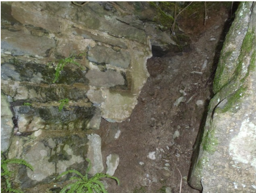
Photo 12 void at upside Blaenau end wing wall 13/02/2014
