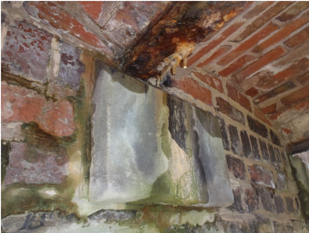
Photo 19 typical water staining at pad stones 13/02/2014
