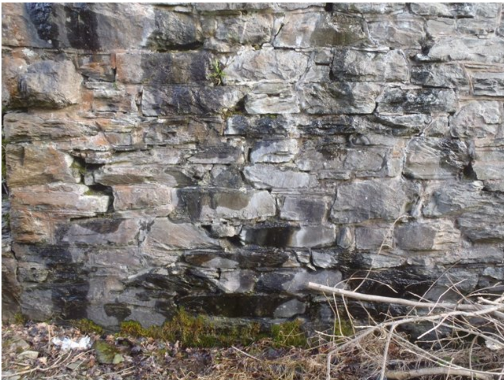
Photo 18 typical water staining at abutments 13/02/2014
