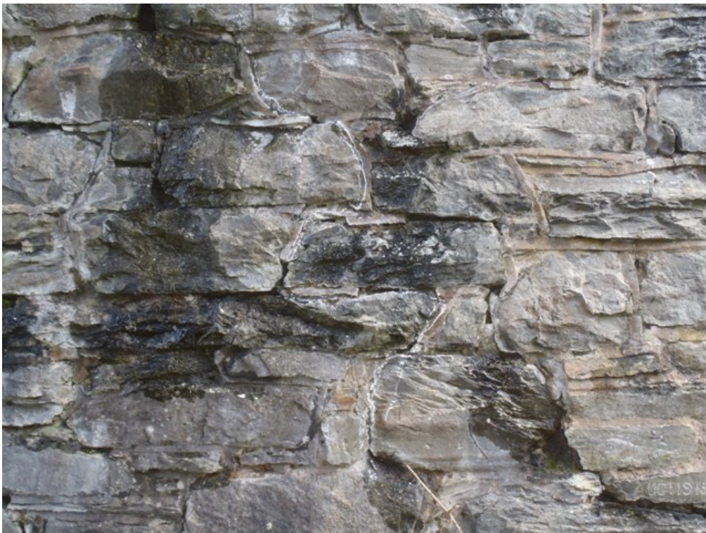
Photo 8 fracture at downside abutment 13/02/2014
