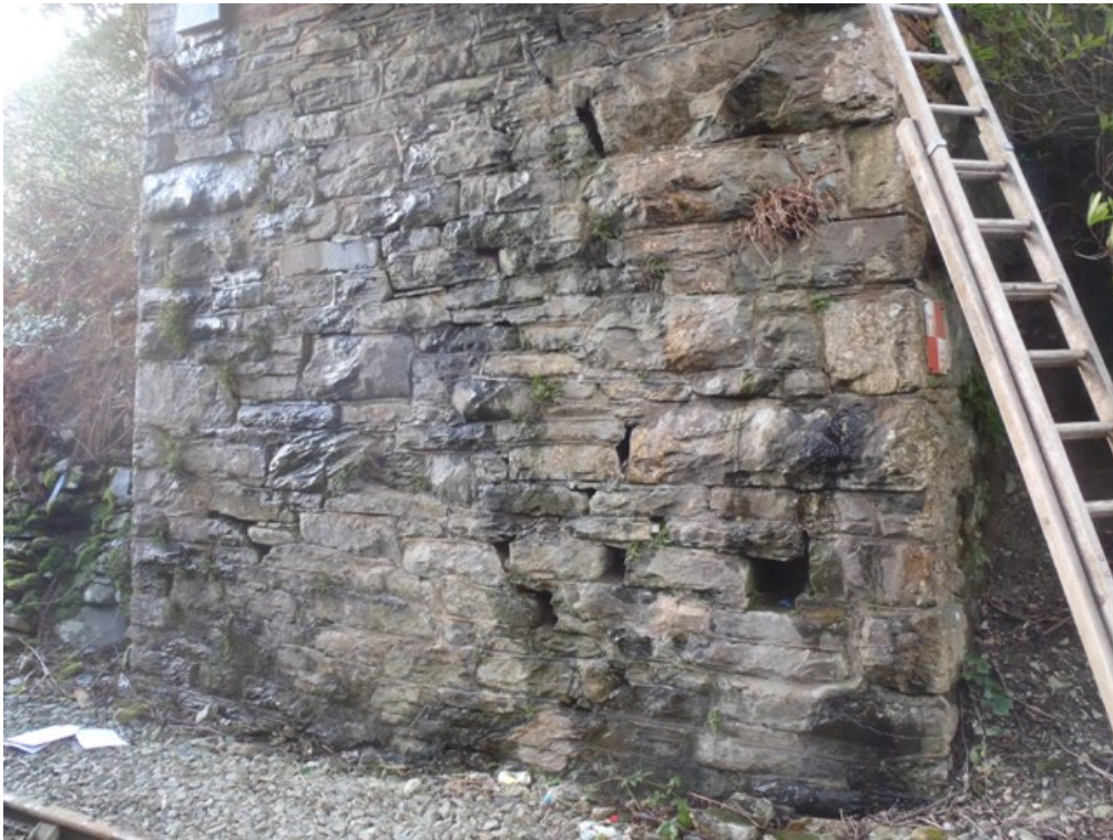
Photo 11 open joints at upside abutment 13/02/2014
