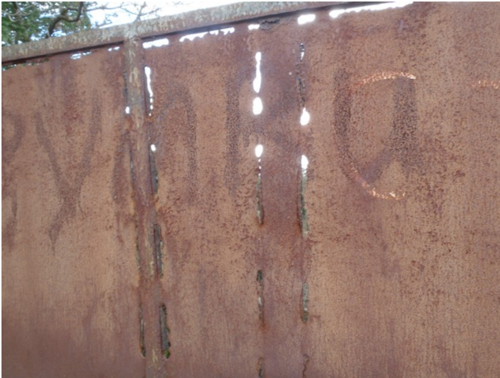
Photo 15 corrosion to Trawsfynydd end parapet 13/02/2014
