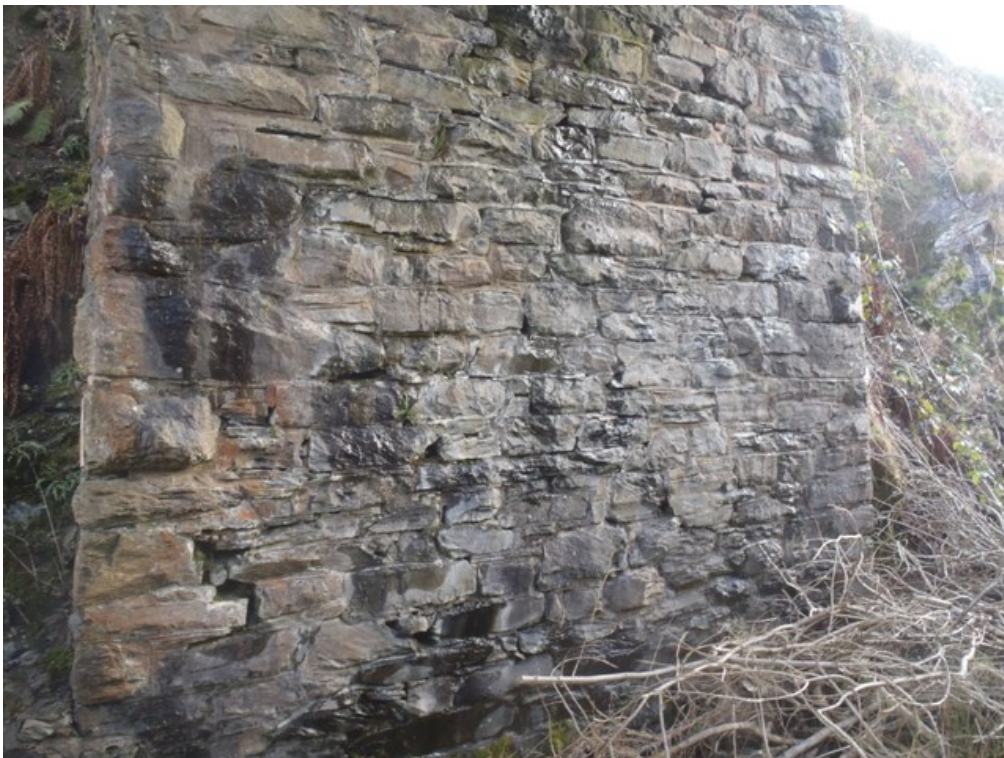
Photo 10 open joints at downside abutment 13/02/2014
