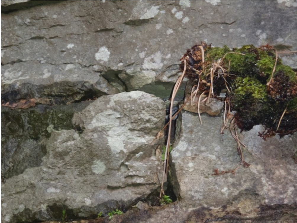
Photo 13 typical open joint at wing walls 13/02/2014
