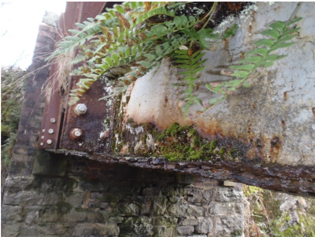
Photo 6 typical corrosion to outer main girders 13/02/2014
