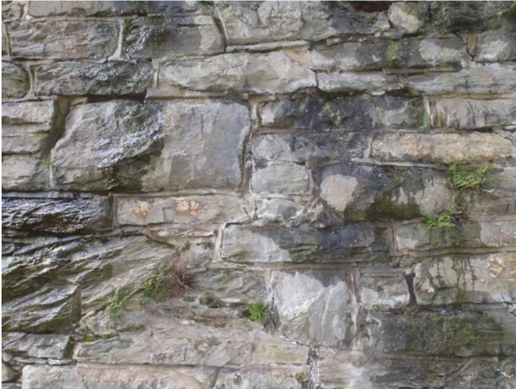
Photo 9 fracture at upside abutment 13/02/2014
