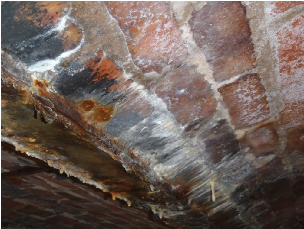
Photo 17 typical water staining at jack arches 13/02/2014
